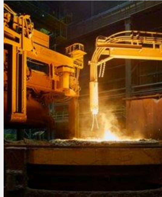
Ladle Refining Furnace Produce Uniform Chemistry and Temp.
